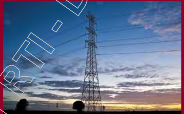
Courtesy of Powerlink
